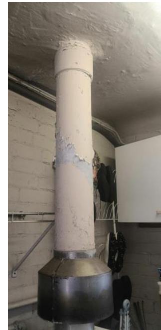
Asbestos exhaust pipe - failed paint coating - friable
