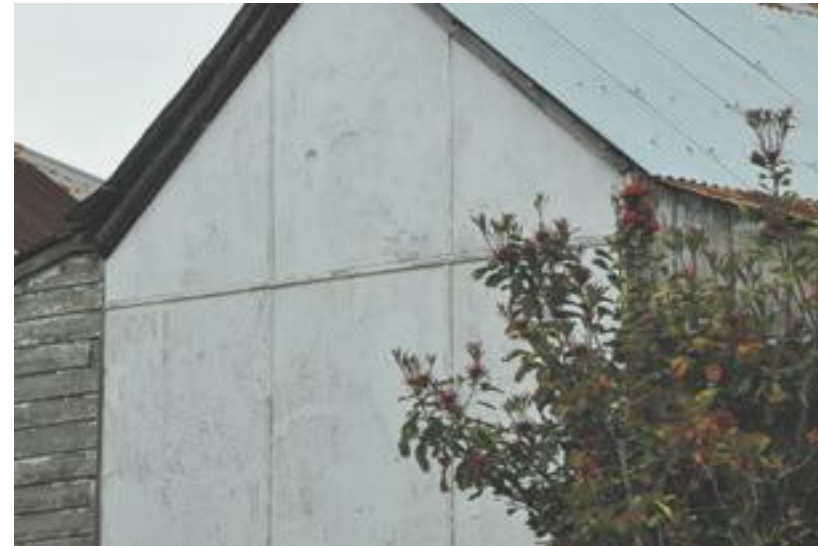
External / internal peeling paint exposing loose asbestos fibres - friable
