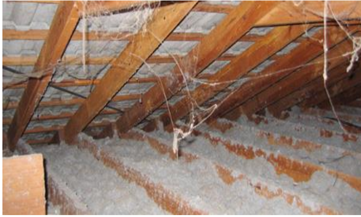
Loose ceiling insulation - friable
