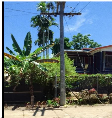
Figure 10 – Electrical power lines connected to project site
